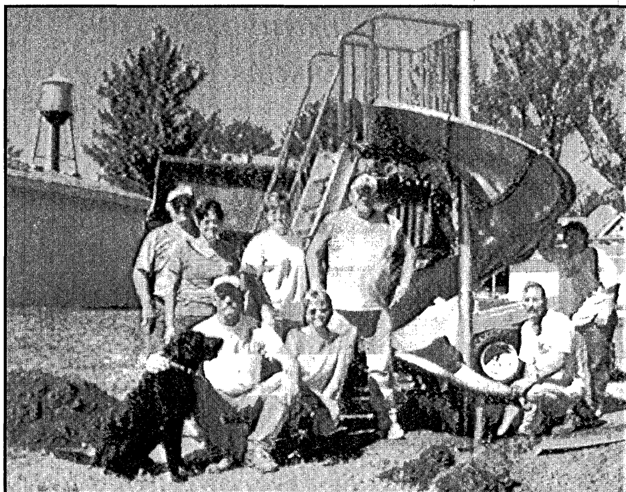
Members of the construction crew pause from their work for a photo. The group worked hard putting in improvements recently at the Concord Village Park in Concord.
